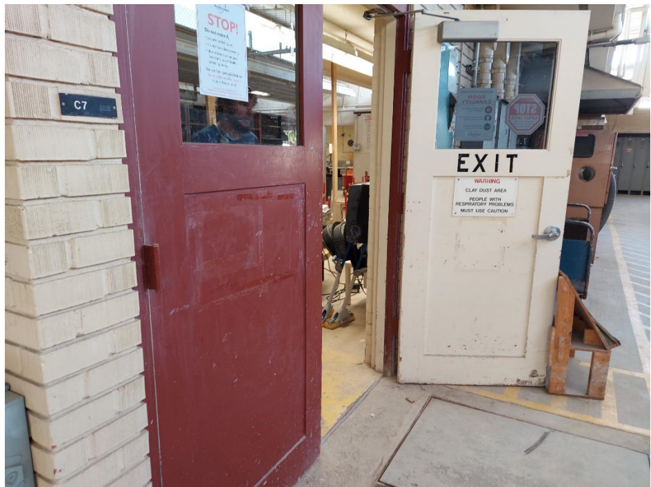
Photograph 10: Tripping/rolling hazard at double door entrance to Room C7.
