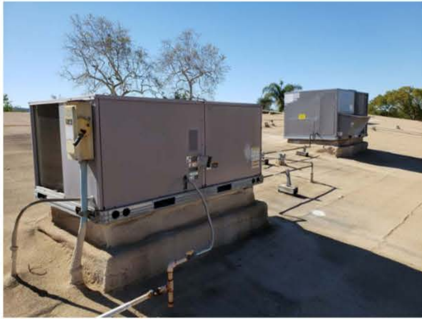
Photograph 1: Two of several SSC roof-mounted air handling units (AHUs).
