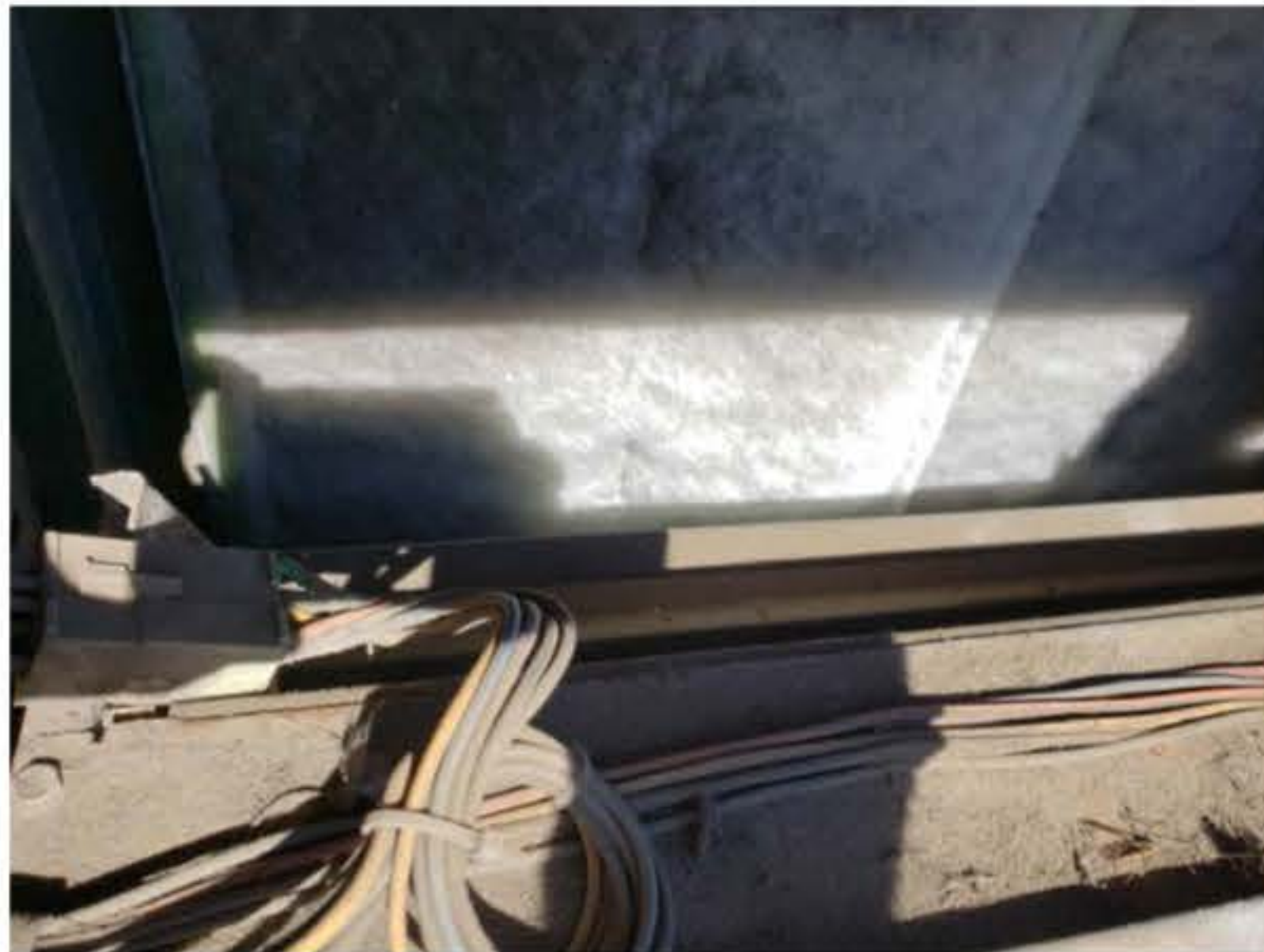
Photograph 2: Interior of SSC AHU showing UL-rated MERV 8 Dacron filters.
