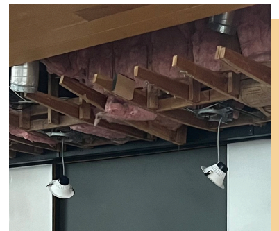
Ceiling damage due to aging building
