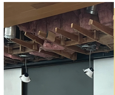
Ceiling damage due to aging building
