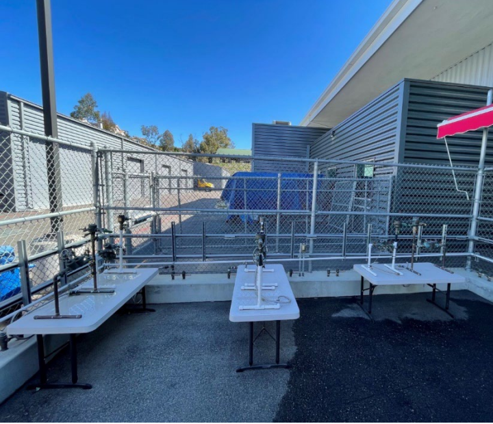
Old backflow units.
