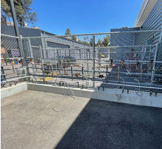
New Backflow Units
