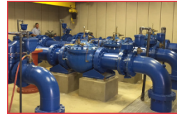
Water Distribution: Operating the entire system of pipes, pumps, motors, valves, and tanks to ensure safe and reliable delivery of water to homes and businesses.
